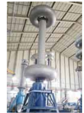
[V-series test termination]
